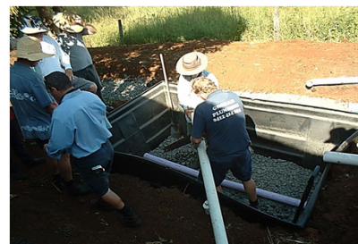
Underdrain and gravel bed
