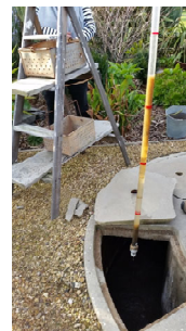
Figure 6: Sludge Depth Test - First Primary Chamber
