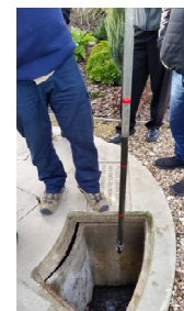
Figure 13: Sludge depth test – Subsequent service
