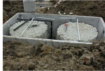
Waterloo Biofilter, Canada
